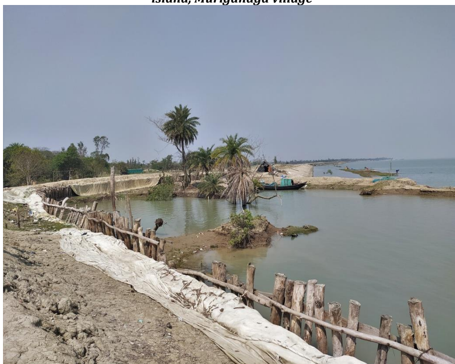
Photo 4.7: Ring embankment constructed after embankment breach and land erosion/loss on Sagar island, Muriganaga village
