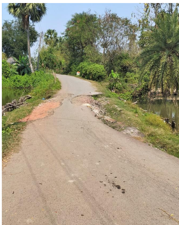
Photo 4.11: Damage of elevated village roads from flooding
